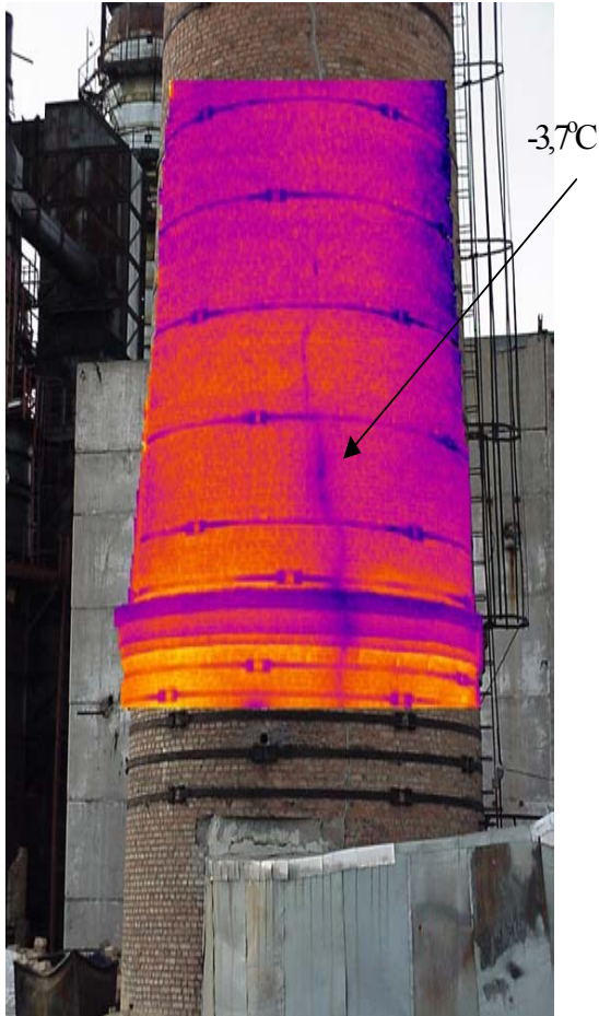
A low quality repair of a through-crack
